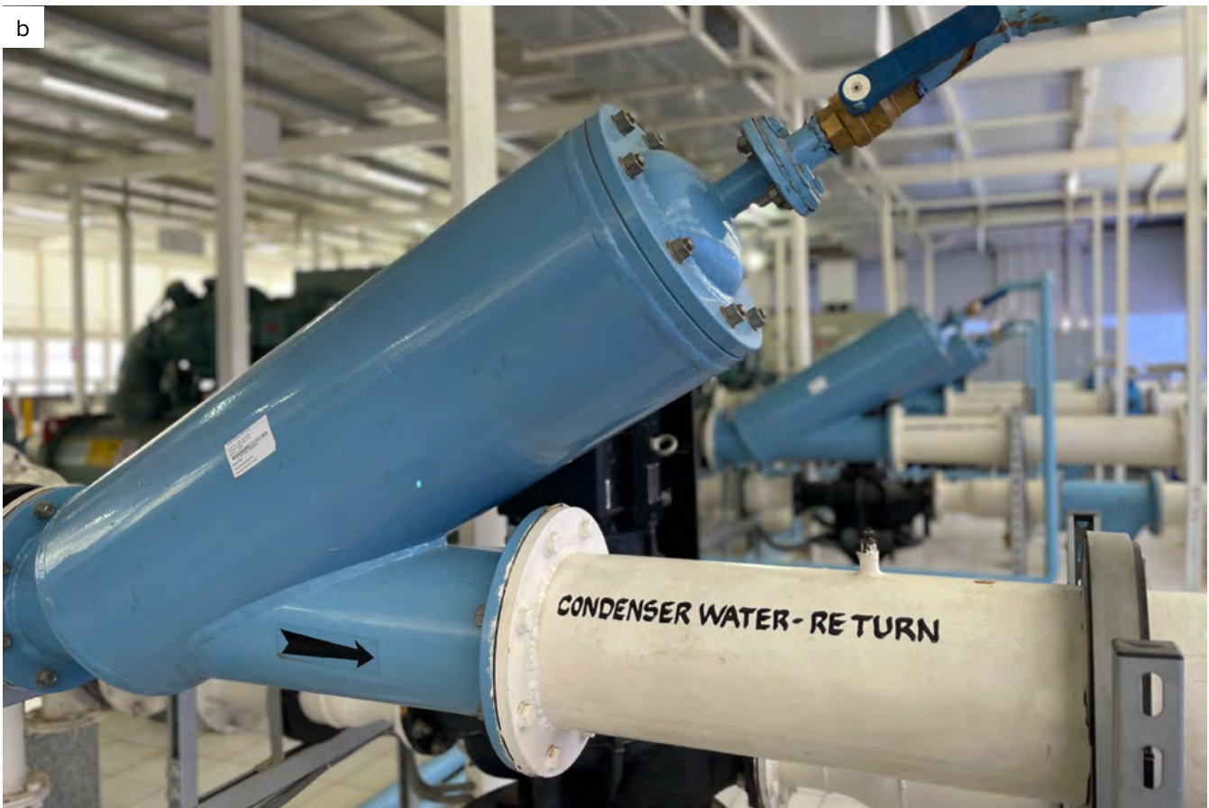
Figure 5.4: (a) Central plant layout, Infosys, Bengaluru, (b) Tube cleaning system on the condenser line
