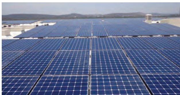
Rooftop solar PV installation, Chennai Mahindra City campus
