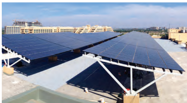
Rooftop solar PV installation, Hyderabad Pocharam campus
