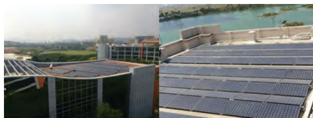
Solar PV installation, Chennai Mahindra City campus
