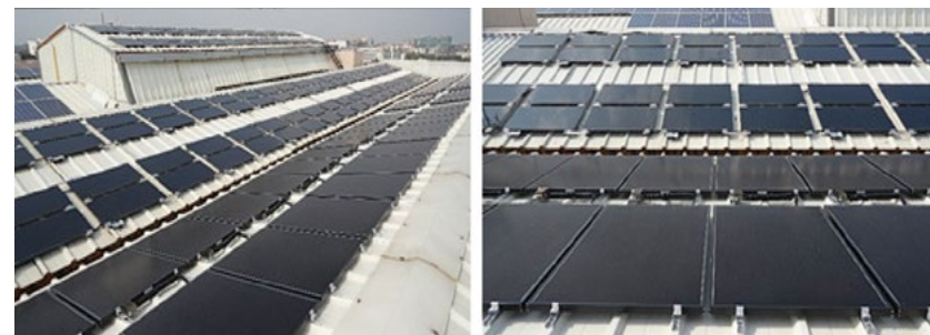
Comparison of different solar PV technologies on the Infosys building rooftop in Bengaluru
