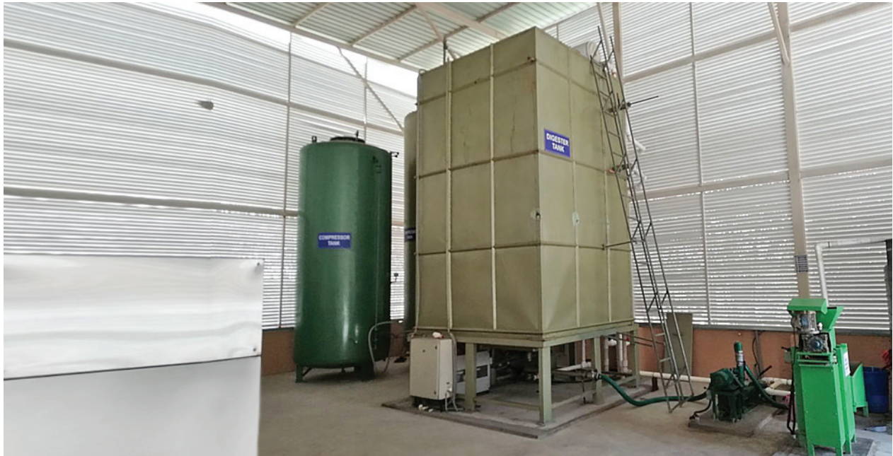
Biogas plant at our Hyderabad campus
