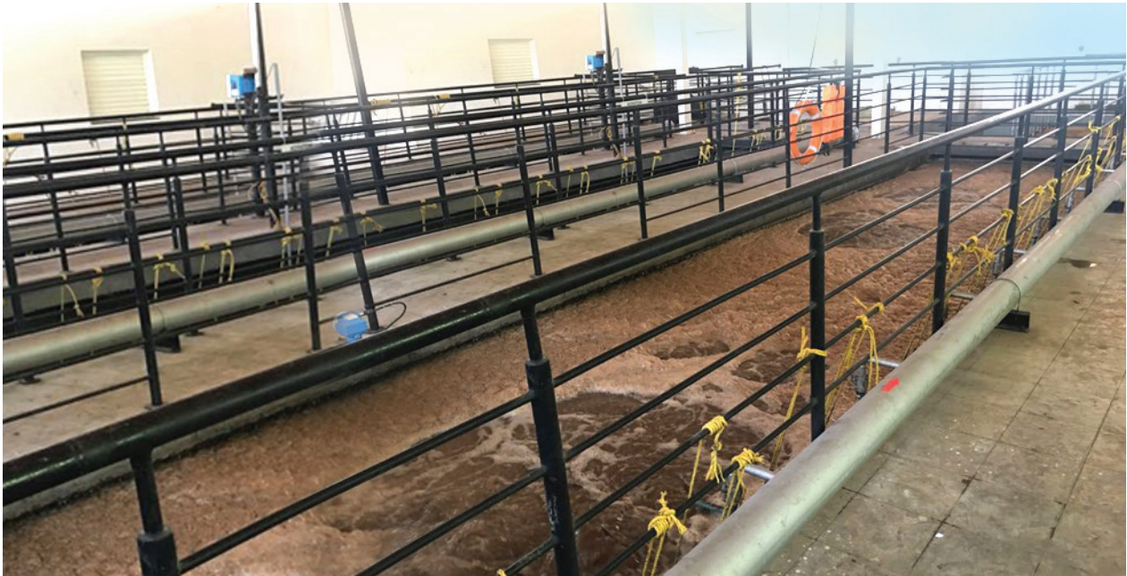
Sewage treatment plant with MBR technology
